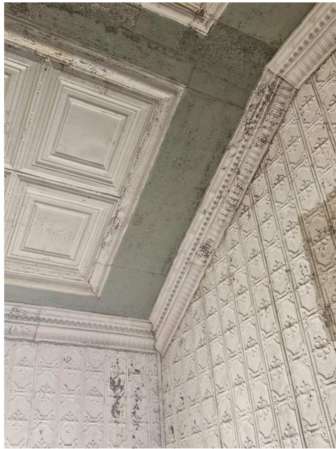
1 EX METAL CEILING TRIM AND TRIM TO REPLICATE ON SLOPED CEILINGS (NORTH AND/OR SOUTH) CONTRACTOR TO REMOVE PANELS CAREFULLY, AND TAKE ALL APPROPRIATE MEASUREMENTS FOR ACCURATE INSTALLATION OF NEW MATERIALS.
