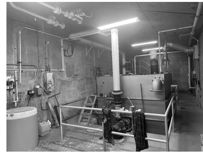
3 West to East Filter Room M100 NTS
